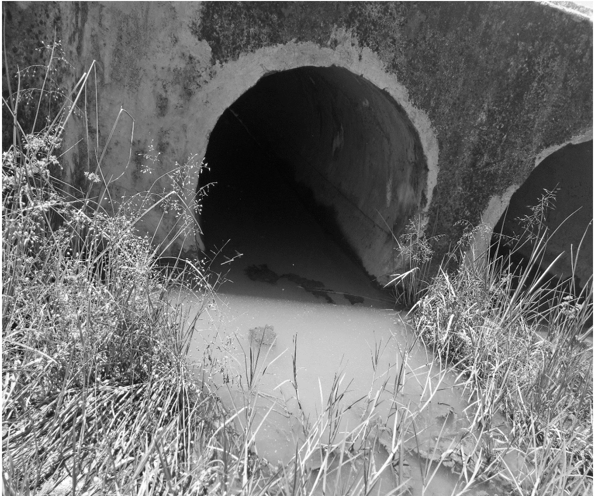
Plate 1.0: Picture of stagnant water under culvert at Lenana Estate in Narok Town Ward.
