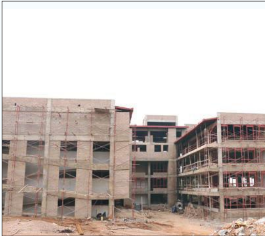
A new home for the university is coming up in Kagarama, Kigali.
